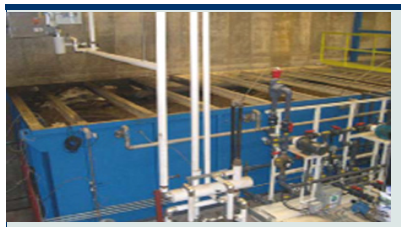
Grey Water Treatment System Convention Center, Pittsburgh, PA
